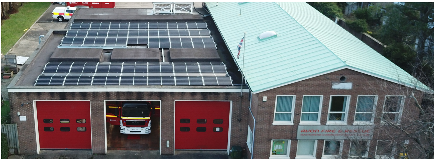
Avon Fire and Rescue Service Clean Energy Project combining solar PV, solar thermal, heat pumps, TEVOLT battery and EV charge points.
